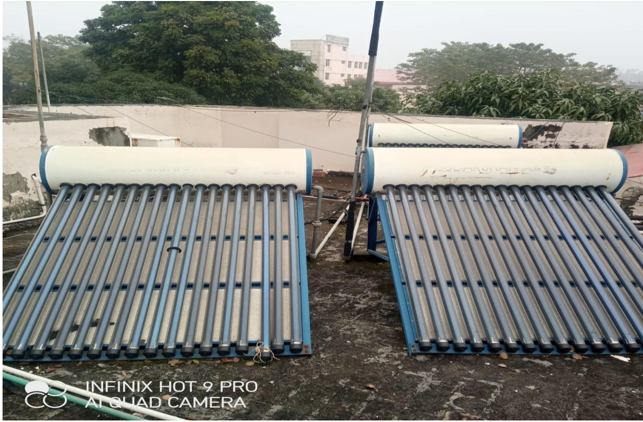
Solar Heater System in the DAVIET campus
