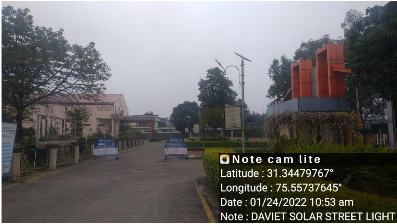
Solar Street Lights installed in DAVIET, Jalandhar
