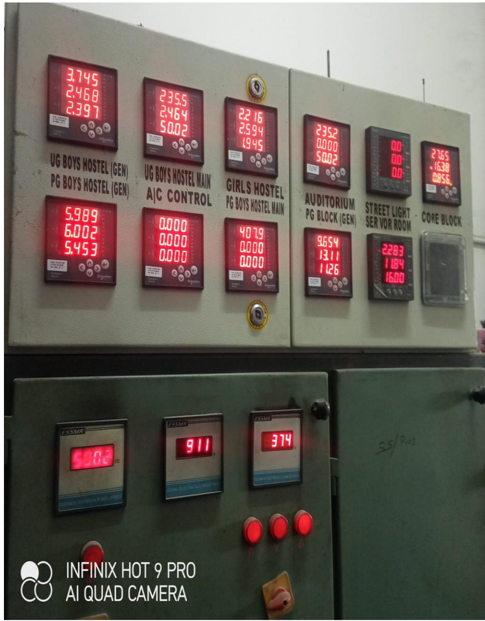
MFM Schneider, Digital meter and CT Current Transfprmaer for the Sensor based energy conservation systems installed in DAVIET, Jalandhar
