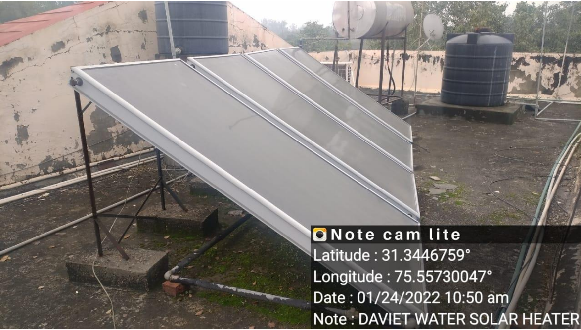
Solar Heater System in the DAVIET campus
