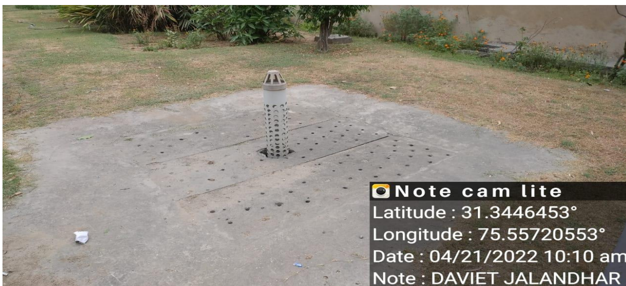
Rain water harvesting system installed in the DAVIET Campus
