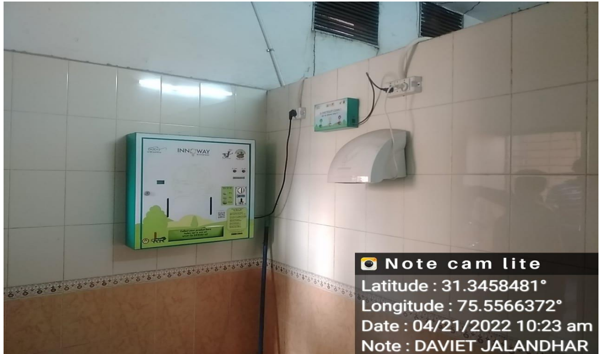
Sanitary Napkin Vending Machine installed in the academic area (core block washroom)
