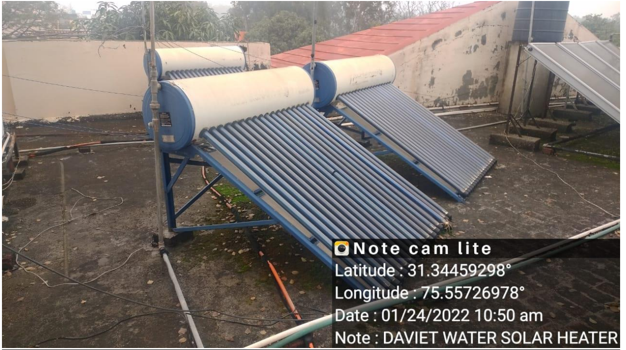
Solar Heater System in the DAVIET campus
