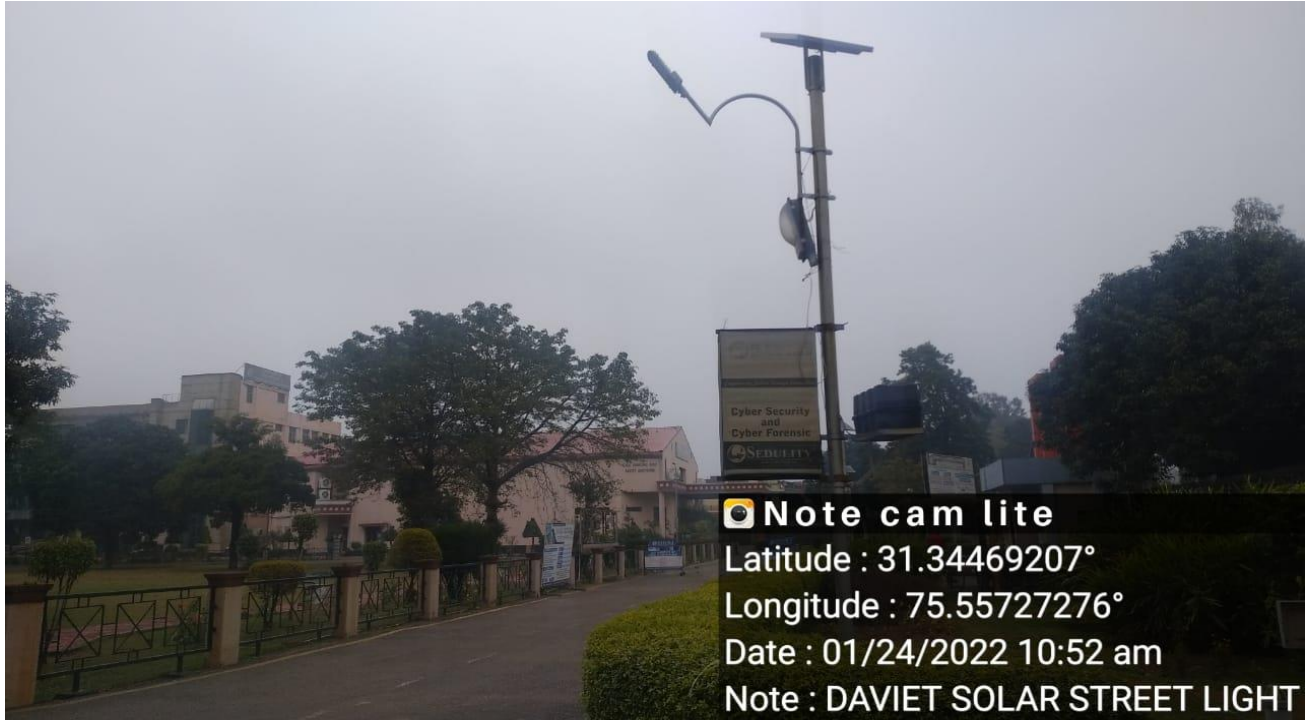
Solar Street Lights installed in DAVIET, Jalandhar
