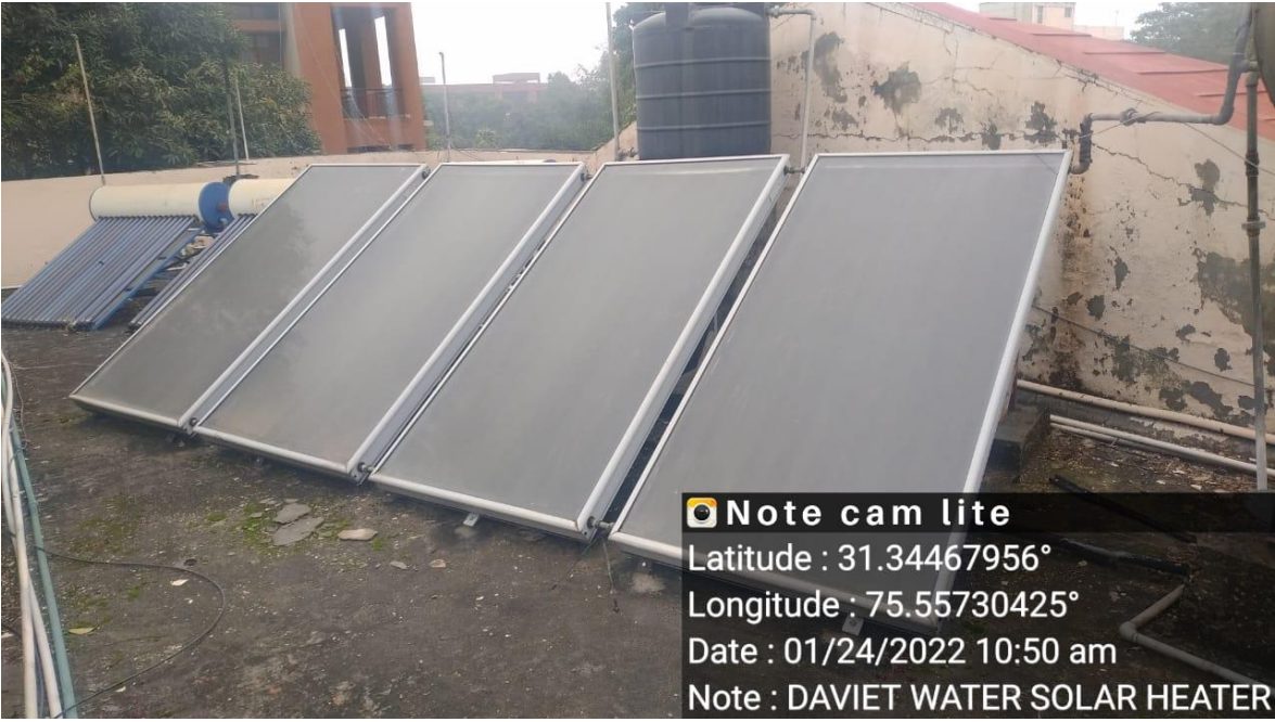
Solar Heater System in the DAVIET campus
