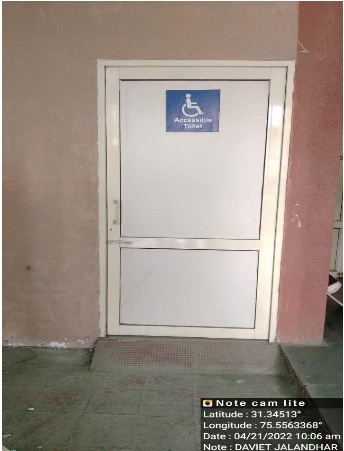
Washroom for Physically Challenged Person in DAVIET
