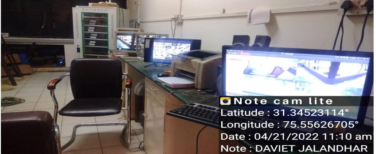
CCTV surveillance Room
